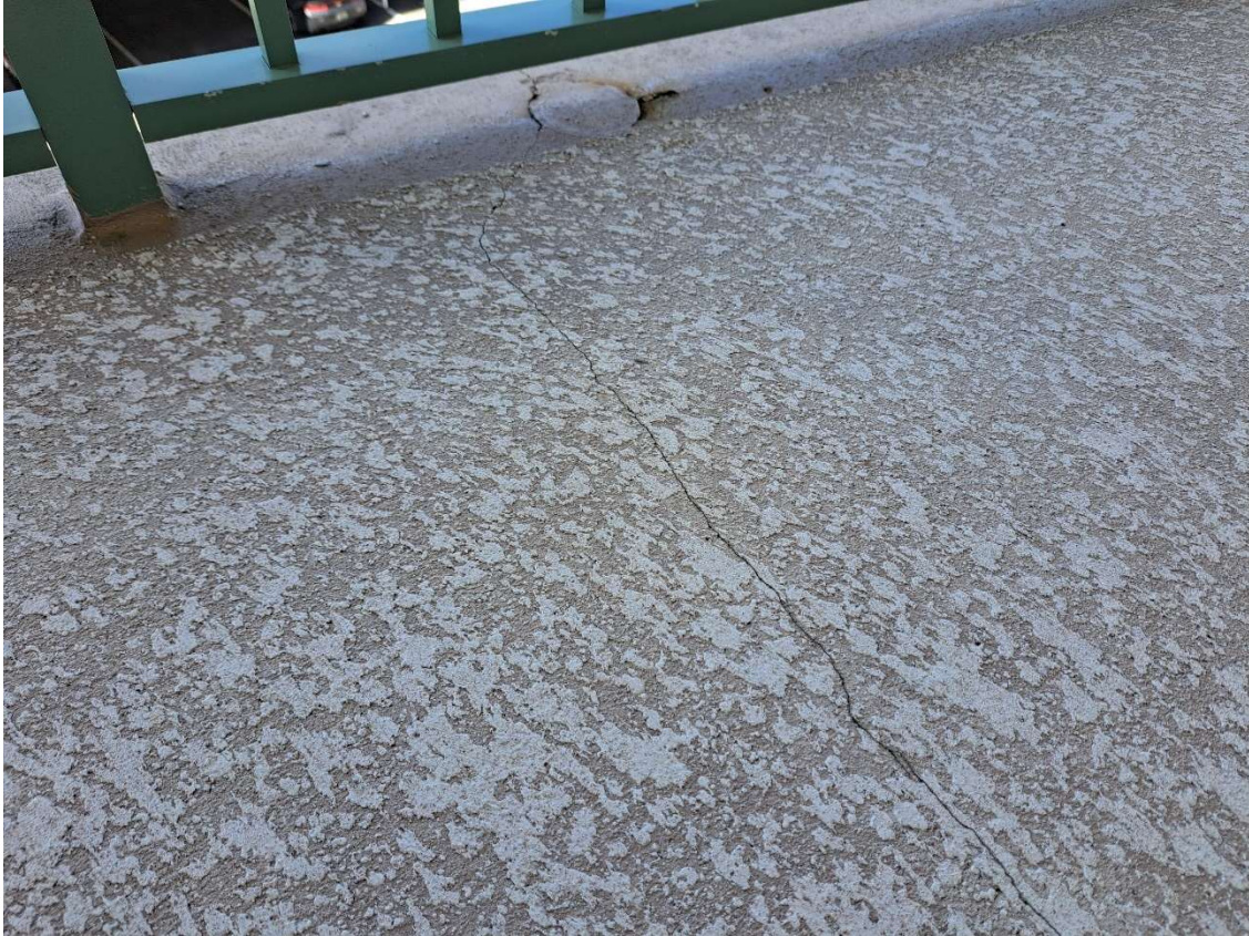
Photo 02 Ref: 2.1.1.1 – Old Post Pockets Causing Cracks On Walkways (Typcial)
