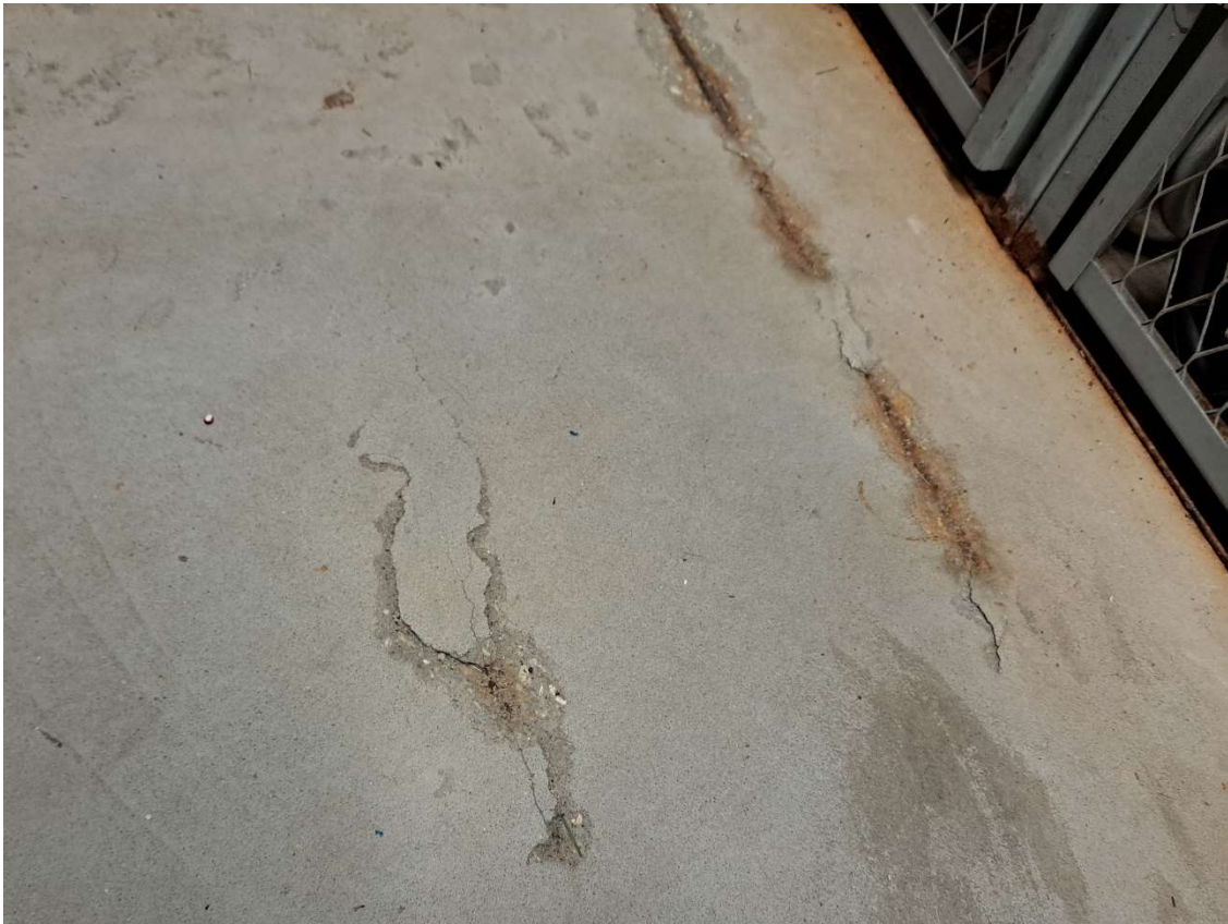
Photo 15 Ref: 2.2.4.1 – Spalling in 4 th Floor Storage Closet Floor
