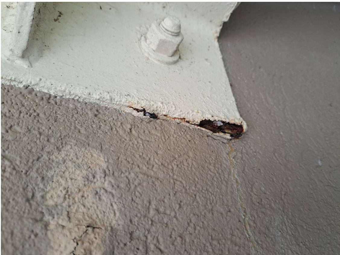
Photo 12 Ref: 2.2.3.1 – Rusting Steel Stair Support Brackets (Typical)
