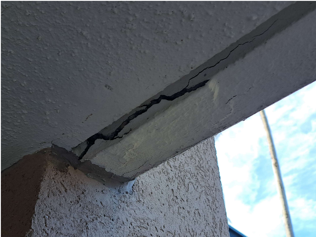
Photo 08 Ref: 2.1.1.1 – Old Post Pockets Causing Spalling and Cracks (Typcial)
