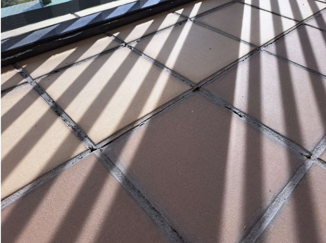
Photo 10 Ref: 2.2.2.1 – Debonded Tile With Damaged Grout (Typical)
