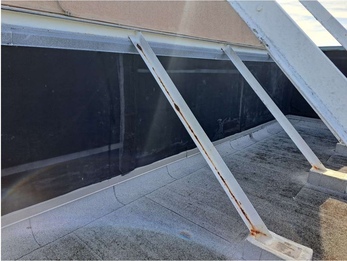
Photo 09 Ref: 2.2.1.1 – Corroded Façade Supports
