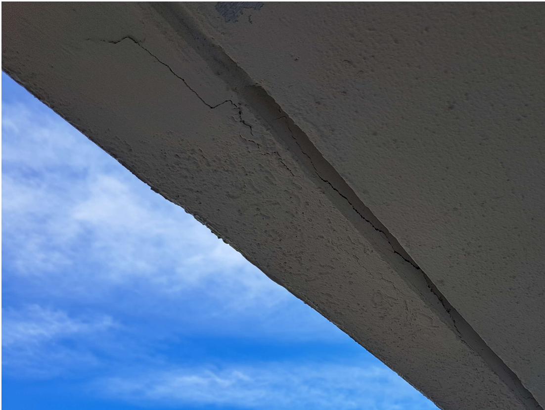
Photo 06 Ref: 2.1.1.1 – Old Post Pockets Causing Spalling and Cracks (Typcial)
