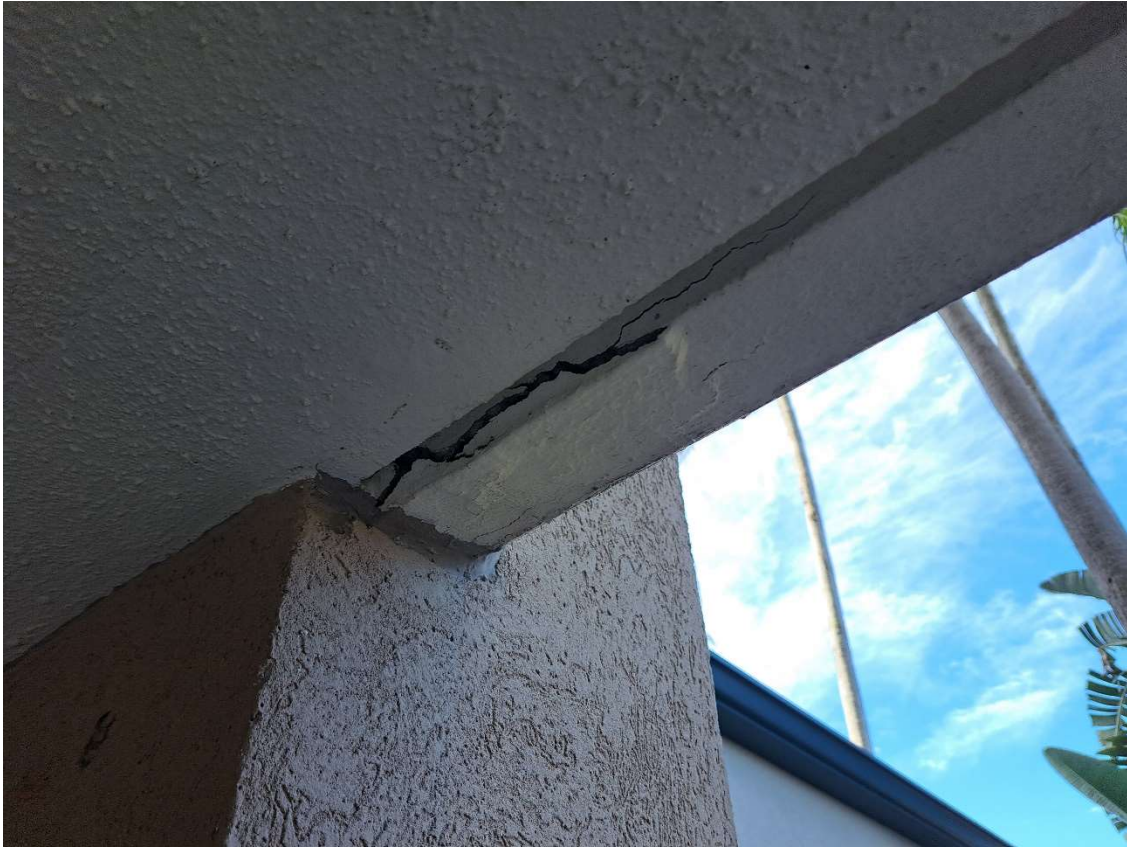
Photo 01 Ref: 2.1.1.1 – Old Post Pockets Causing Spalling On Slab Edges (Typcial)
