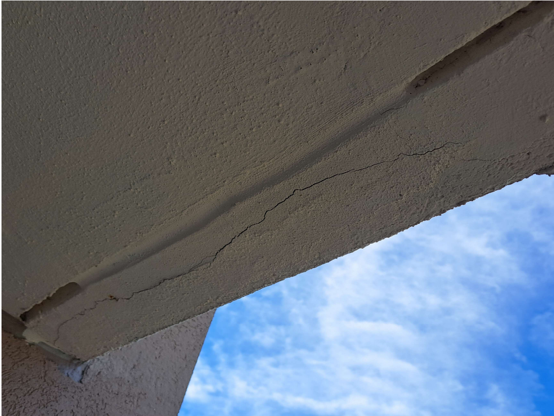
Photo 07 Ref: 2.1.1.1 – Old Post Pockets Causing Spalling and Cracks (Typcial)
