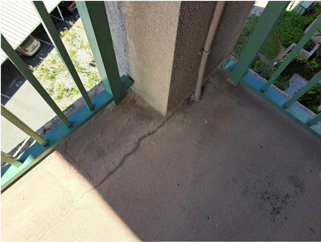
Photo 13 Ref: 2.2.3.2 – Stairway Cracks Along All Landing Slab Edges (Typical)
