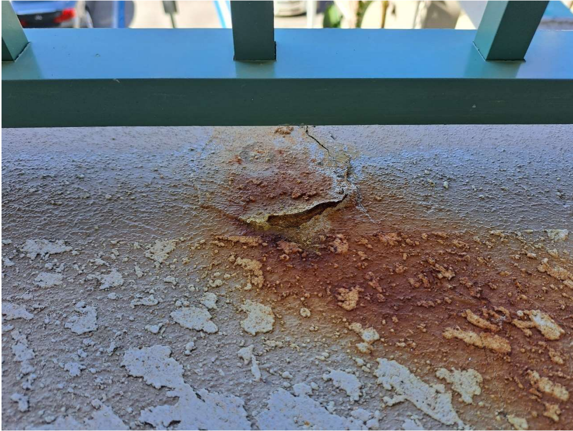
Photo 03 Ref: 2.1.1.1 – Old Post Pockets Causing Spalling Above Post Pockets (Typcial)
