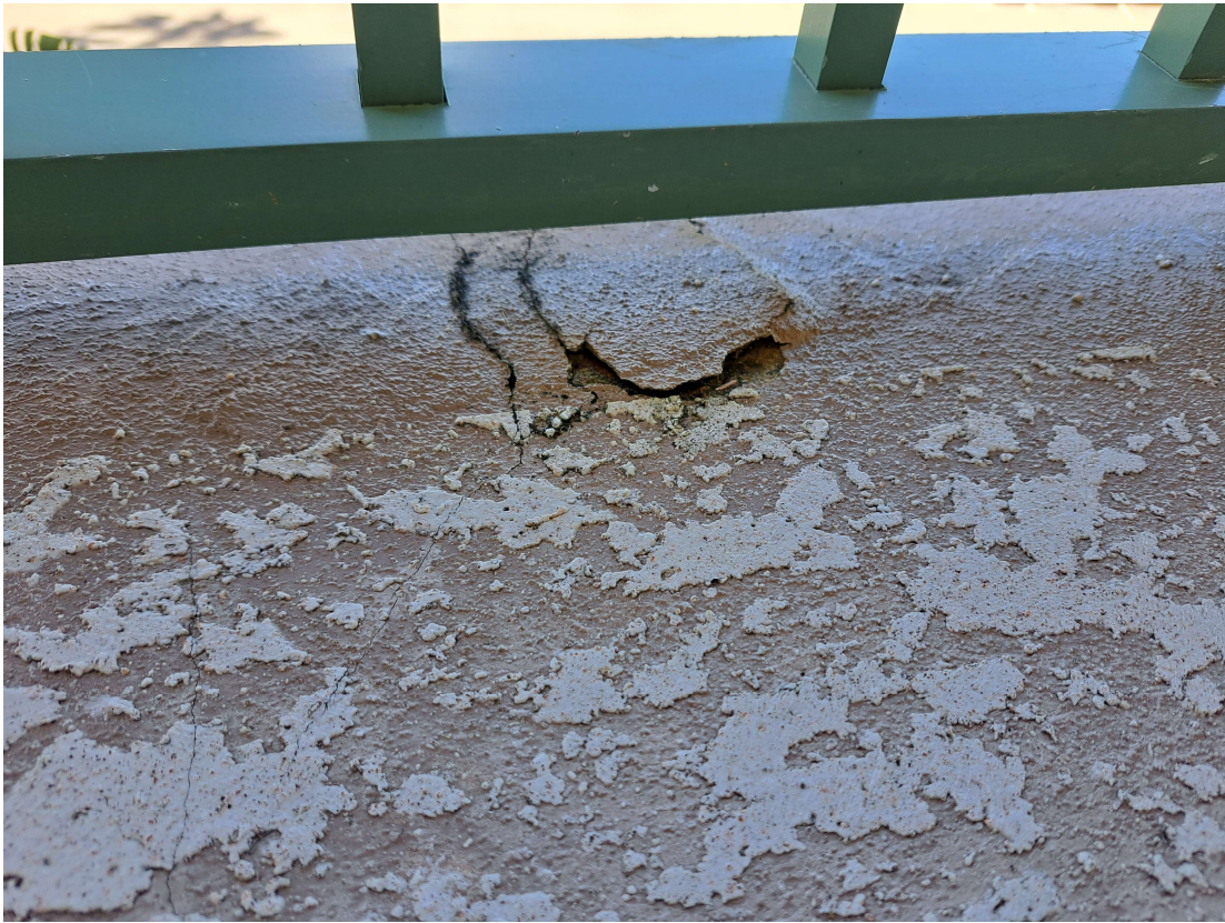
Photo 05 Ref: 2.1.1.1 – Old Post Pockets Causing Spalling and Cracks (Typcial)
