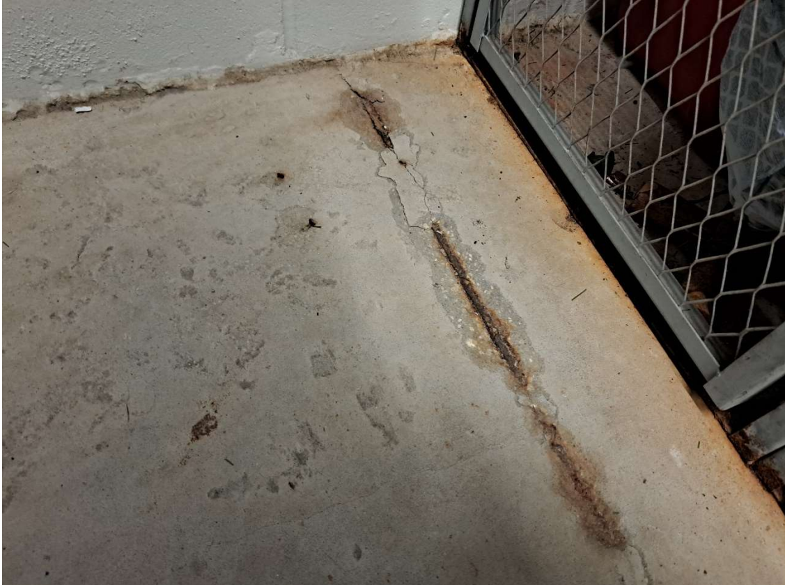
Photo 16 Ref: 2.2.4.1 – Spalling in 4 th Floor Storage Closet Floor
