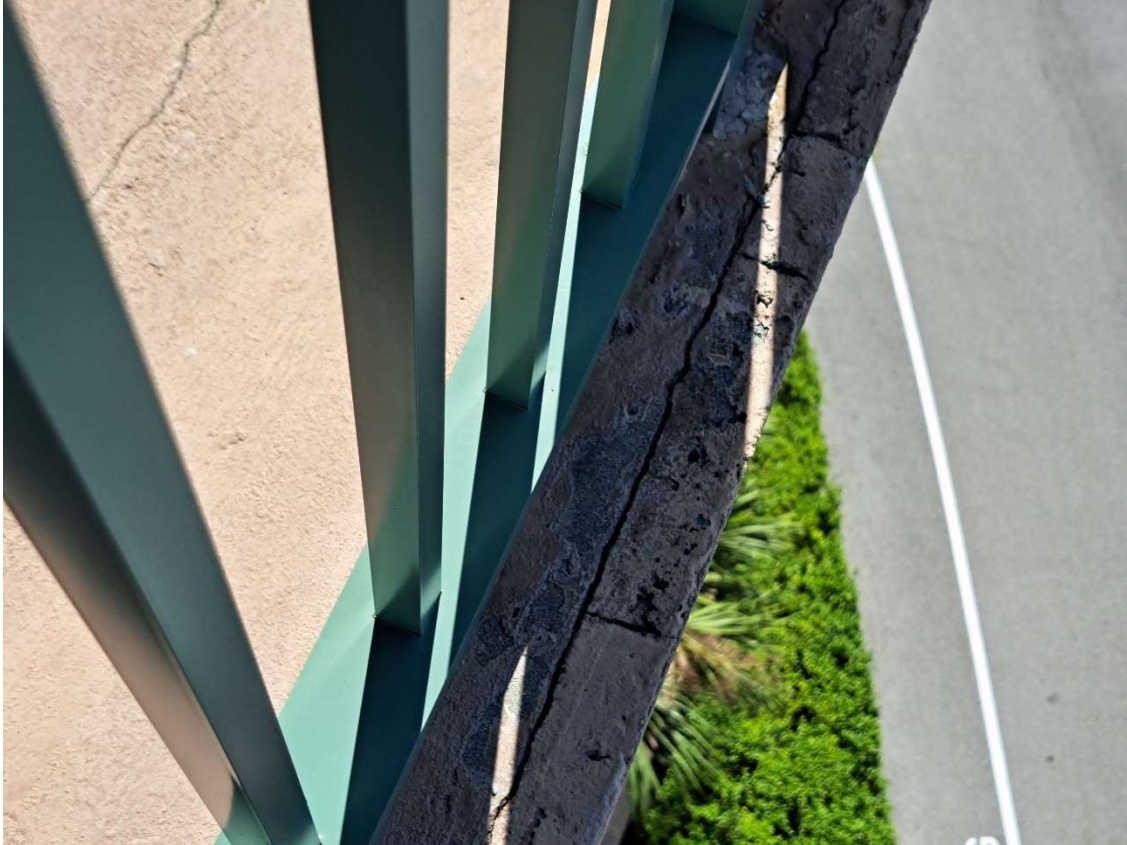
Photo 14 Ref: 2.2.3.3 – Stair EIFS Trapping Water (Typical)
