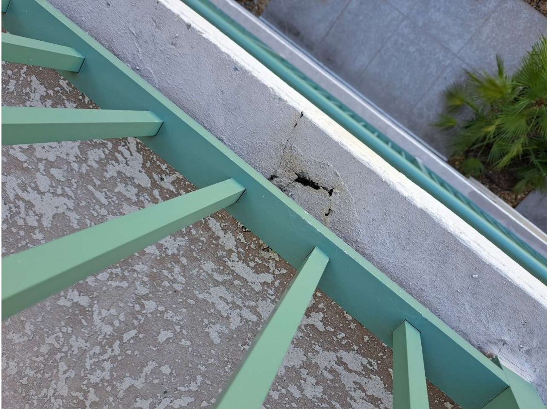
Photo 04 Ref: 2.1.1.1 – Old Post Pockets Causing Spalling and Cracks (Typcial)
