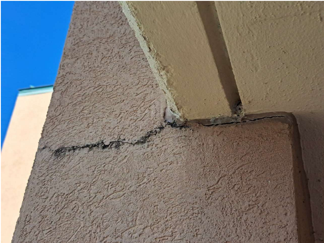
Photo 17 Ref: 2.2.5.1 – EIFS Trapping Water (Typical)
