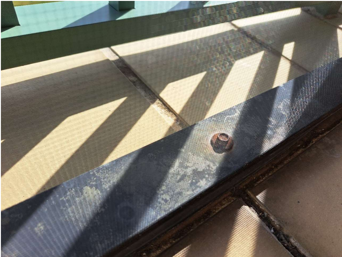
Photo 11 Ref: 2.2.2.2 – Corroding Screen Enclosure Fasteners (Typical)
